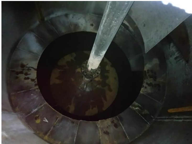
Figure 21. Feedwell (inside view).
